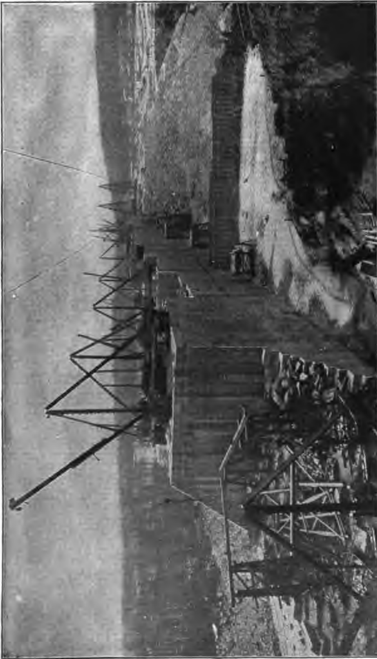
PLATE 42.—View of Construction of Olive Bridge Dam, Showing Derricks, Cableways, Cyclopean and Concrete Block Masonry, and Transverse Joint in Dam.
